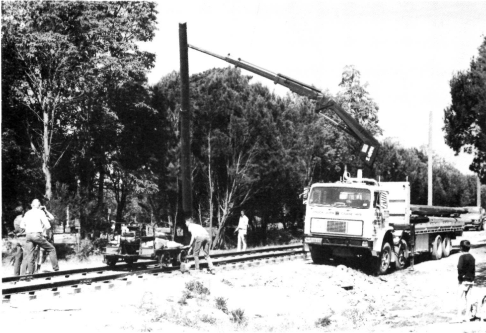
Erecting poles along the main line. Sixteen poles were set on Saturday, 12 September 1987.
