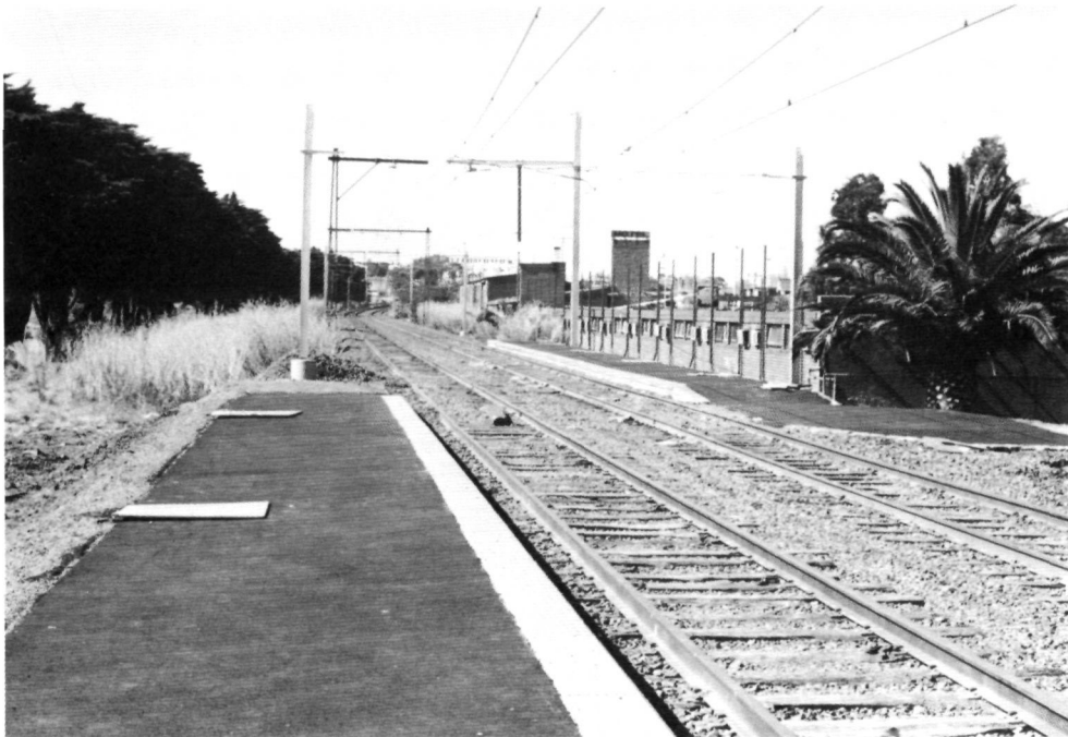
This additional stopping place is being constructed between St Kilda and Middle Park. The staggered platforms still require lighting and fencing (and some form of shelter). The added overhead stanchions can also be seen in this view.
