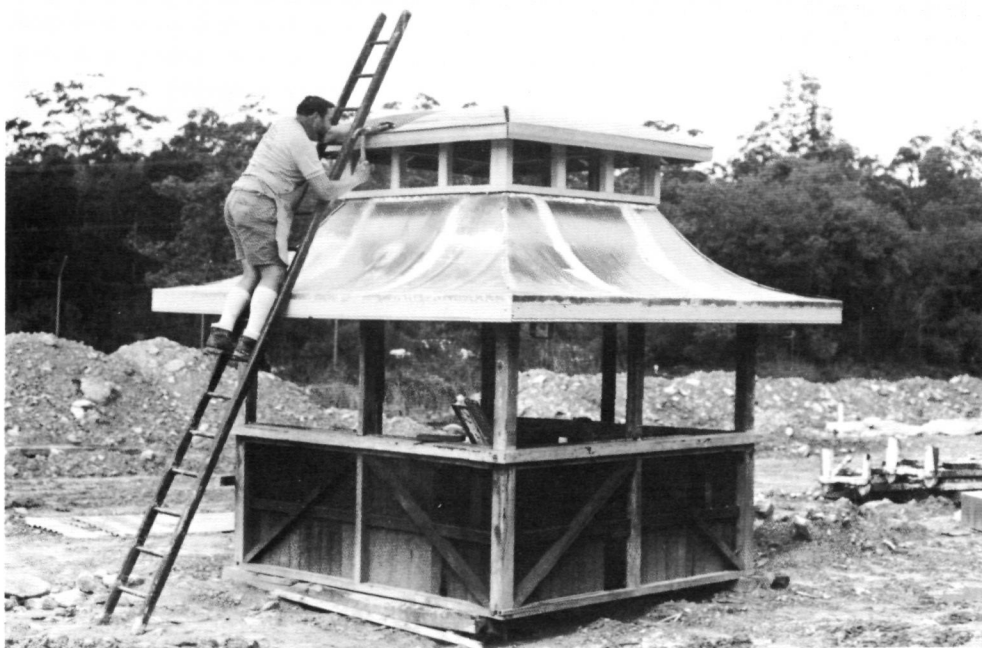
Derek Butler at work on the re-roofing of the signal box from the Railway Square Waiting Shed on 15 August 1987.
