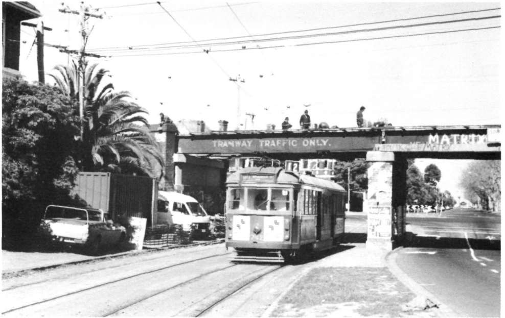
This bridge over Albert Road will carry the LRVs over the St Kilda Beach routes (Routes 10 and 12) tramway and the opportunity is being taken to carry out needed repairs to the structure.
