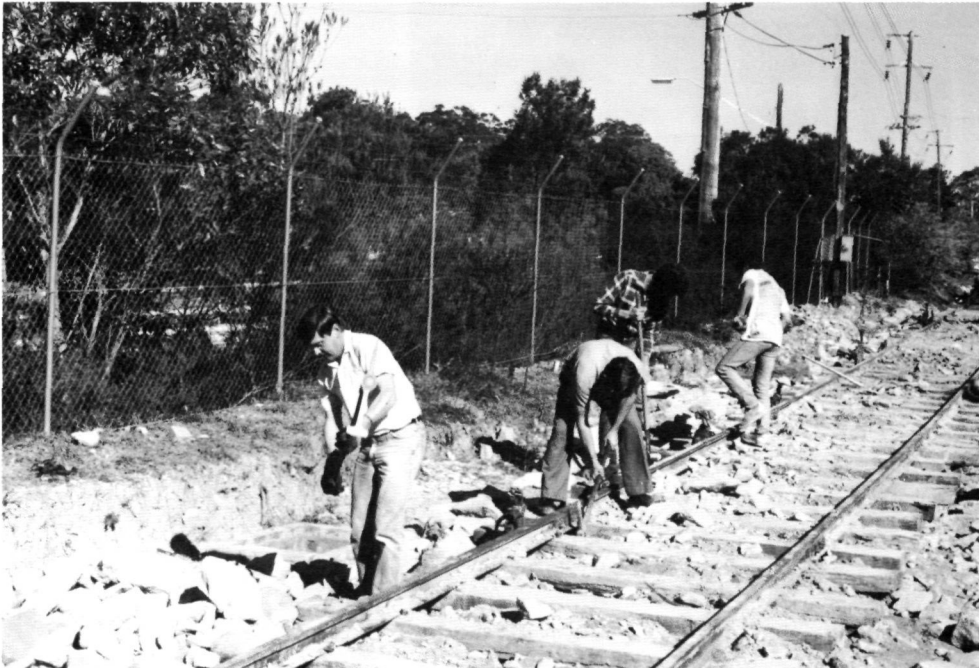
Trackwork from Pitt Street to the scissors crossover was completed during August/September 1987.
