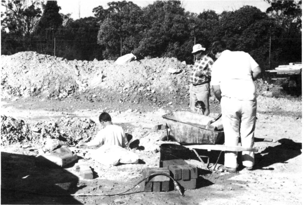
Putting down drainage pipes and constructing sumps is an important part of the construction work. Here a sump is being bricked in the future Lakewood Park area on 12 September 1987.
