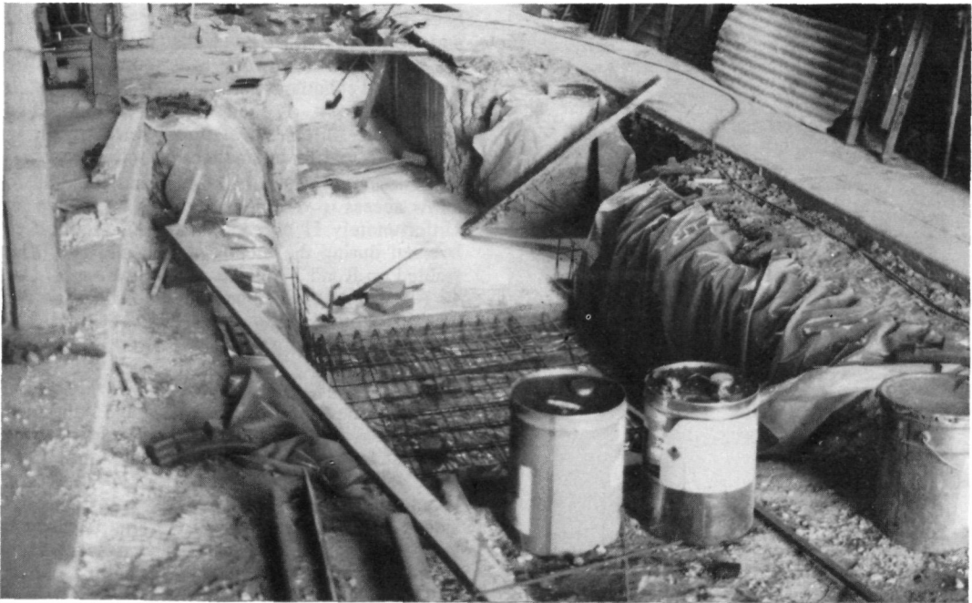
The cement floor for the western pit extension was laid in two stages. The section in the centre of the photo has been laid while wire mesh for the second section is in place.
