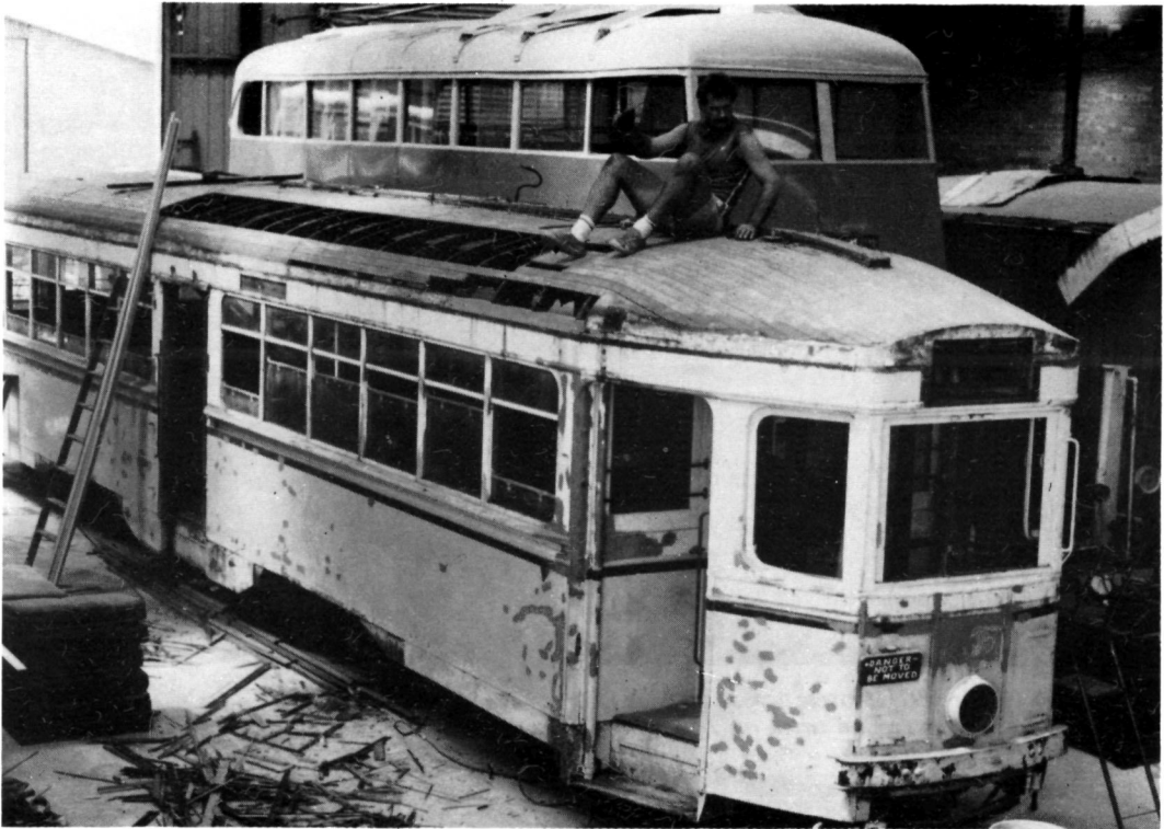
R1 class 1971 undergoing roof repairs in the workshop. The fascia on the visible side of the car has been removed and coachbuilder Geoff Spalding is replacing rotted and damaged roof boards.
