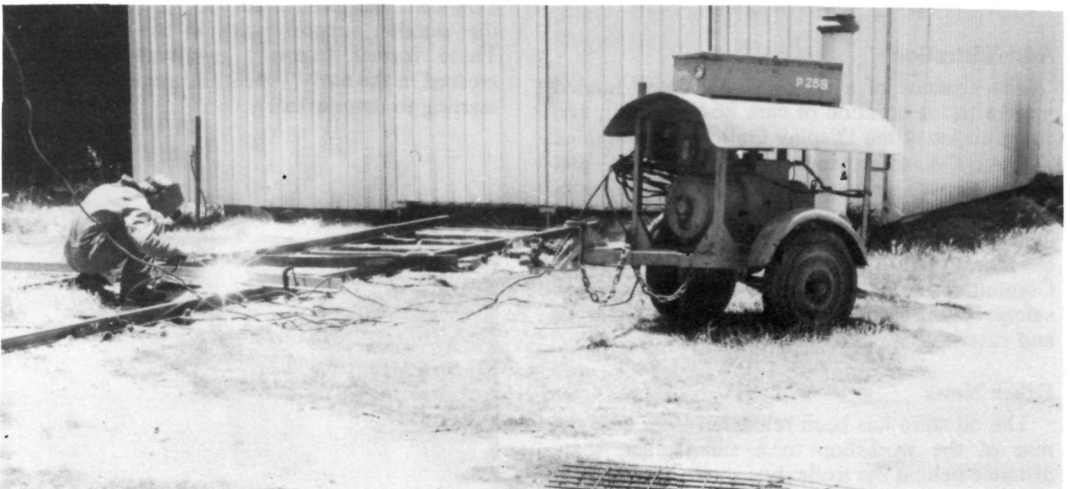
Ian Seymour uses one of our ex-MTT 600 volt DC portable tramway welders to weld a length of angle iron used to repair one of the main depot support poles.
