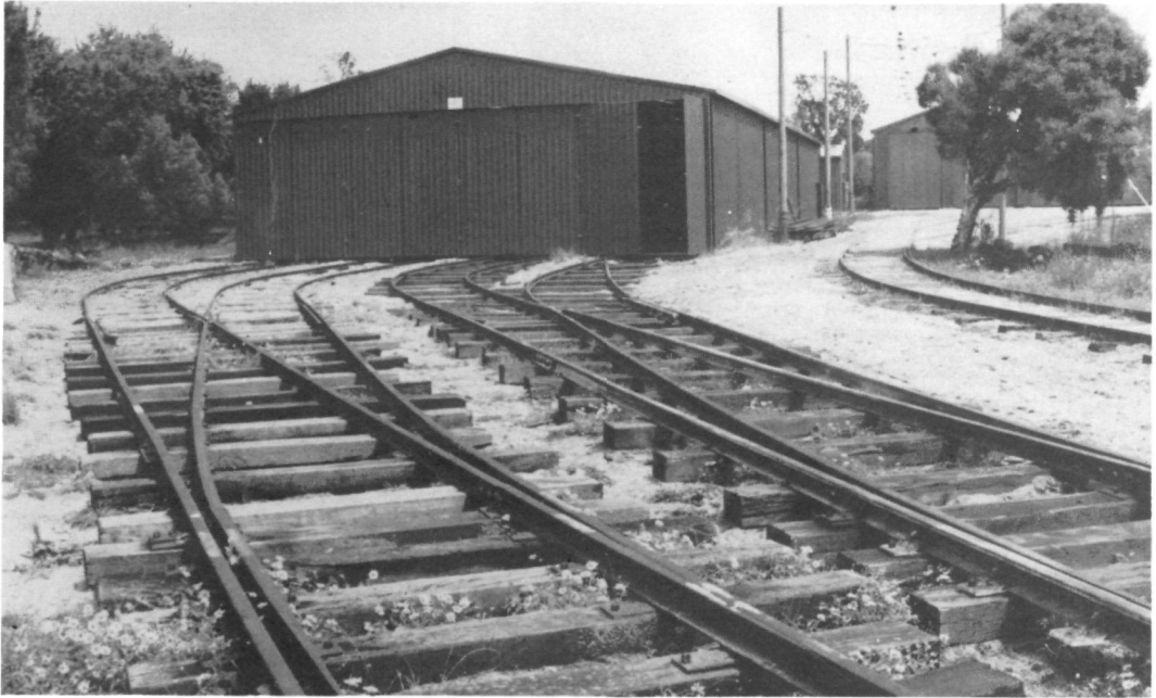
Tracklaying on the new fan for the tram body storage shed was almost complete on 18 October 1989. The rail at right remains to be spiked.
