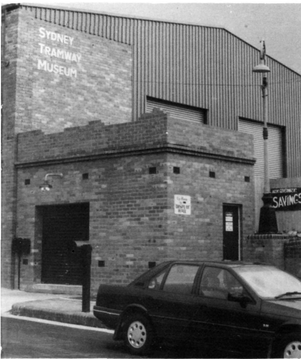
The permanent office for our traffic staff is being constructed above the substation building, the roof of which was designed to be the floor of the new office.
