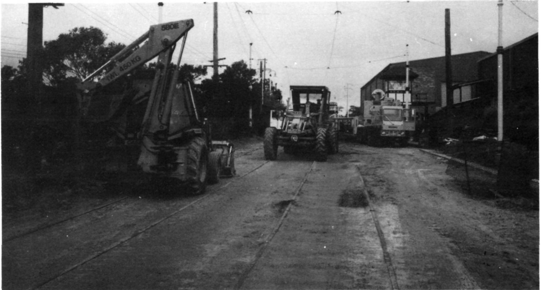
Sutherland Council's earthmoving equipment prepared the street for the laying of roadbase which was compacted over ensuing weeks in preparation for the hotmix sealing.
