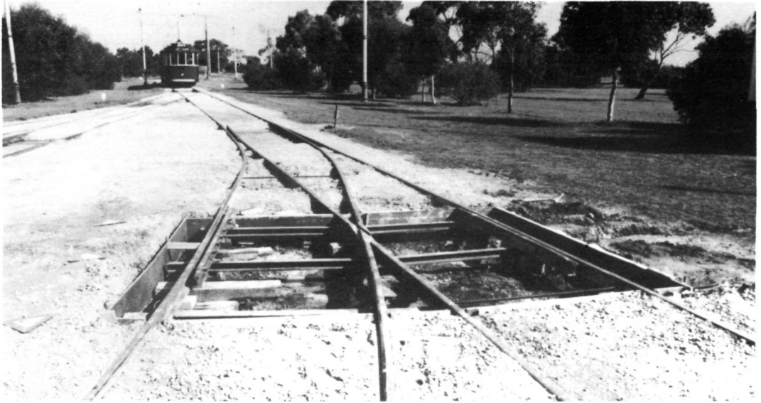
The new Roads 2/3 crossing has been boxed ready for concreting. Car 264 in the distance is about to enter the depot fan.
