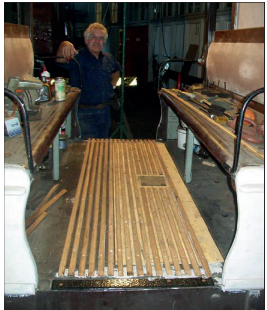
One compartment floor of the double-deck car has been completed, with floor slats and the access plate fitted over the opening to the bogie pin. Member David Lewis admires his efforts.
