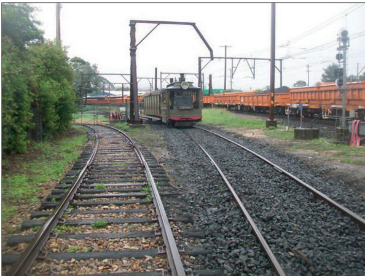
Motor 103A and car 93B venture onto the new track, laid where there were previously two disused turnouts. The train on the adjacent track at right was being used for spent ballast removal during a shut down.
