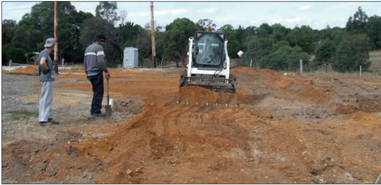
Daniel Edwards and Anthony Smith assist our local bobcat contractor in levelling the site for the Lower Terminus and new shed. Jacqui Smith
