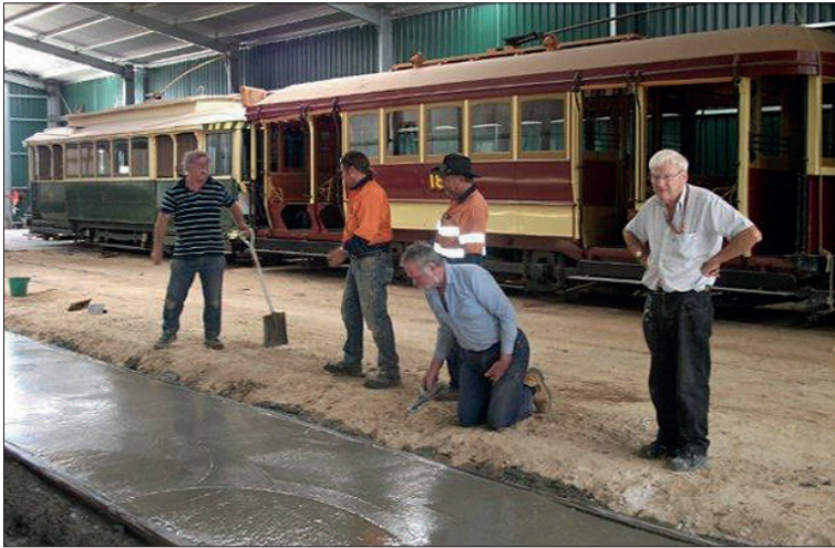
The AETM gang at work on the second concrete pour on 18 January. Chris Summers
