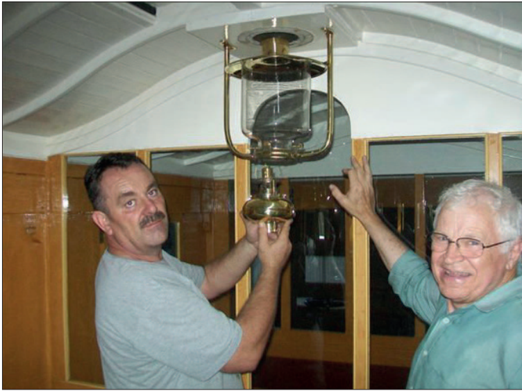
Craig Connelly (left) and Bruce Irwin (right) installing one of the lamps in tramcar 93B.
