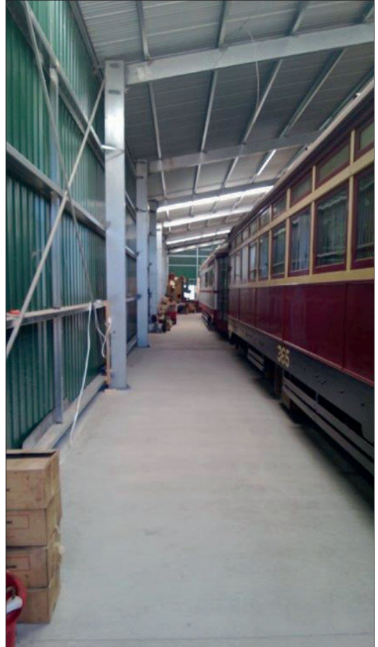
The concrete aisle between Road 4 and the northern wall of the new Mechanical Maintenance building was poured and laid by a contractor during the last week of February.
