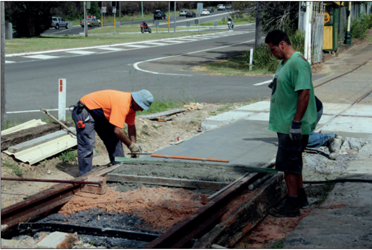
Danny Adampoulos finishes off a load of donated concrete on 23 April, assisted by Scott Aston and a CSO worker (hidden).
