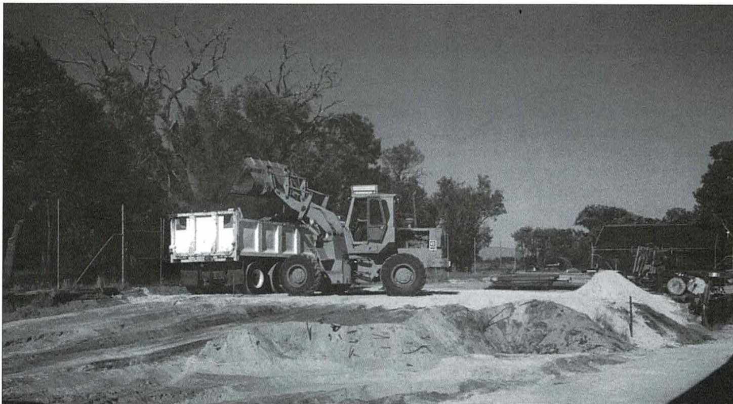
Excavation and levelling of the site for the spare parts storage shed, November 1995.
