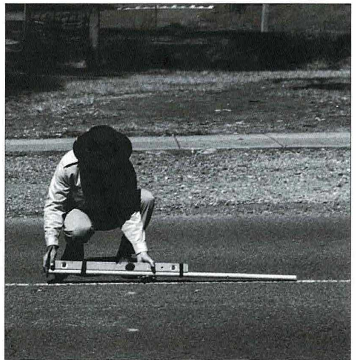
John Lambert measures the fall (slope) of the road surface at the proposed level crossing in Tramway Street outside the museum.
