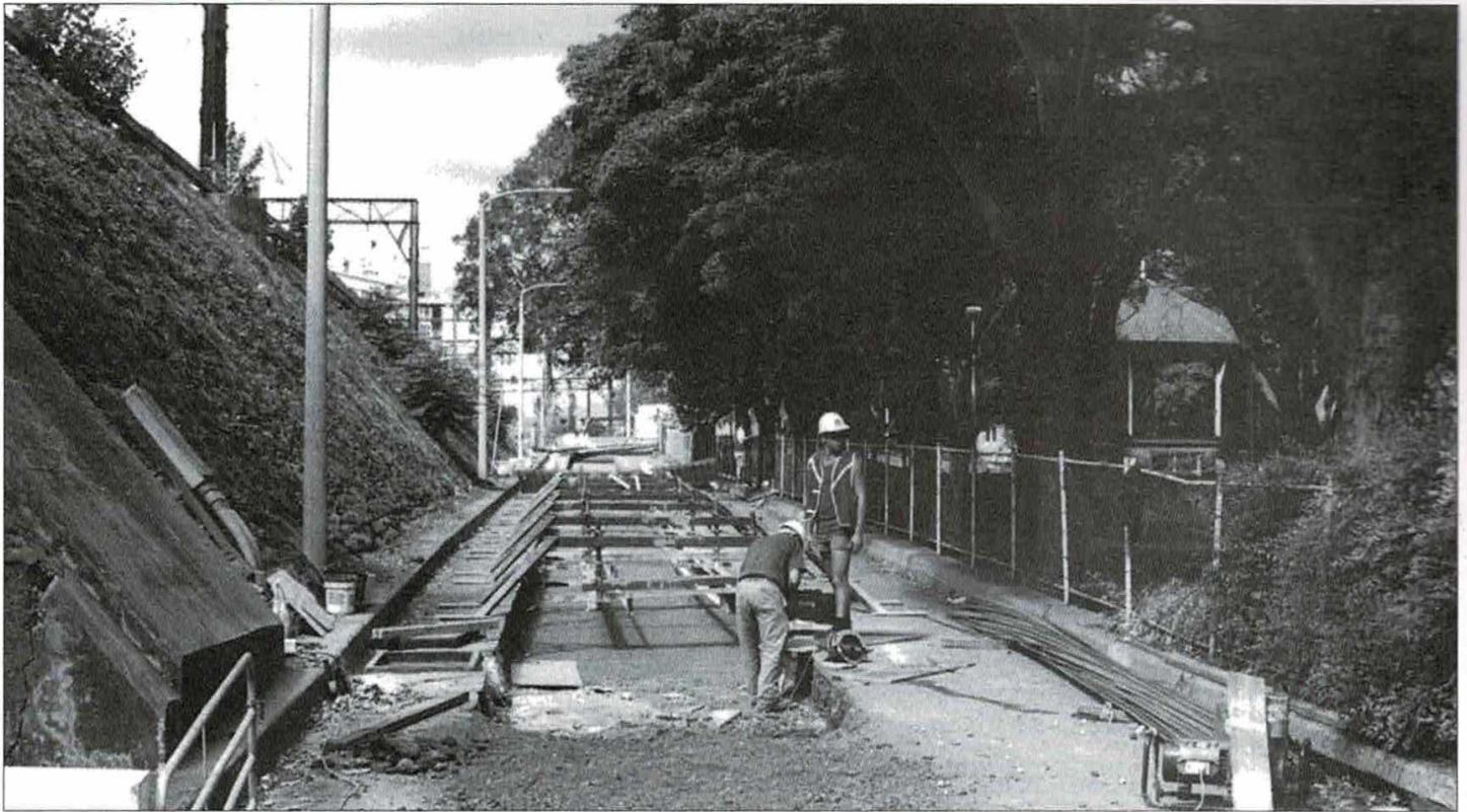
Construction of the concrete roadbed up the eastern ramp to the railway colonnade on 23 March 1996.
