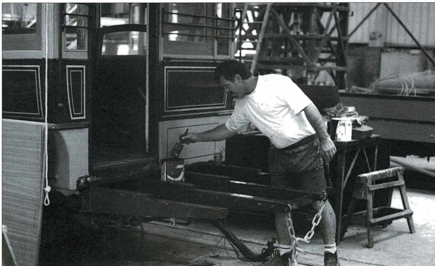
Geoff Spaulding primes the platform bearers at the No.1 end of C class 290.
