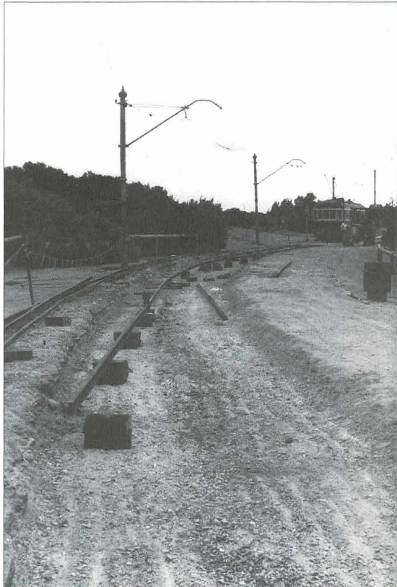
This view of the playground curve track excavation looks back to the temporary playground terminus where works car W2 354 waits.
