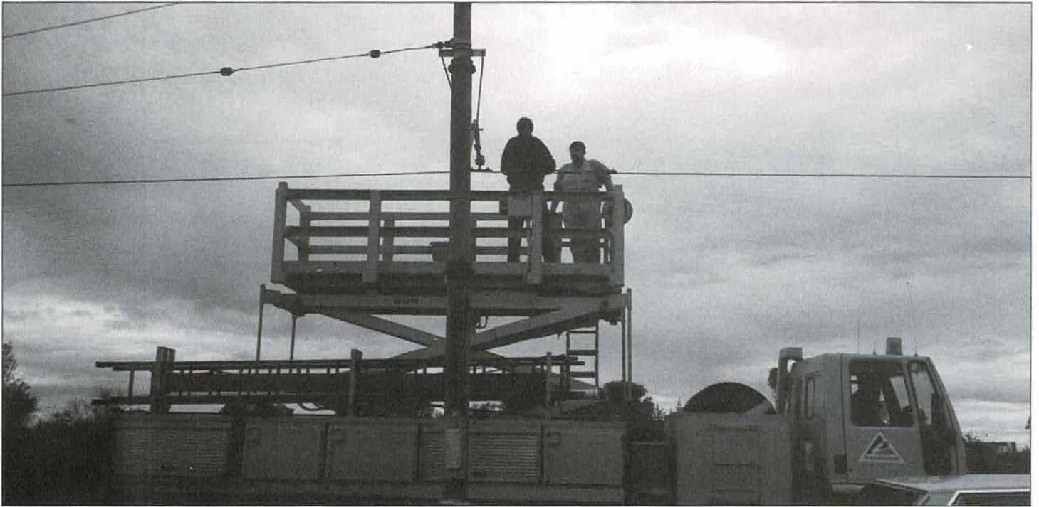
Dave from TransAdelaide and Kym Smith restore the overhead wire at pole 46 using the TransAdelaide overhead truck. This is the pole from which the new wire was run to the beach terminus on Friday 28 June 1996.
