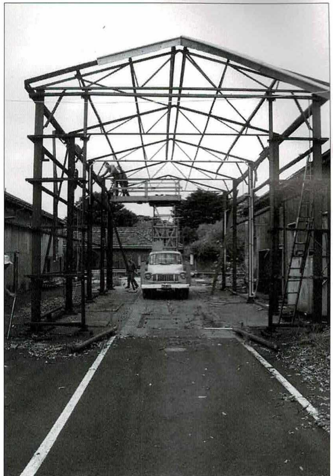
The Tramway Museum Society of Victoria dismantled the former bus wash building at Elwood Depot. In this view, the dismantling is well under way with roof and side sheets already removed.
