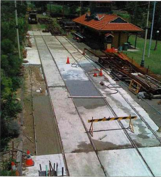
An aerial view of the Railway Square track relaying work in November 2010. It is taken facing south, and shows the completed western track and areas to be completed.
