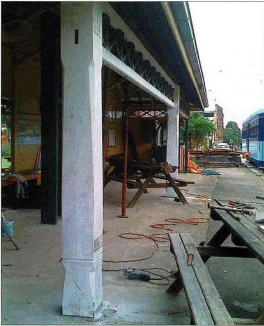
The two new columns and truss have been installed on the Railway Square waiting shed. Work continues to secure the roof to the truss beams.
