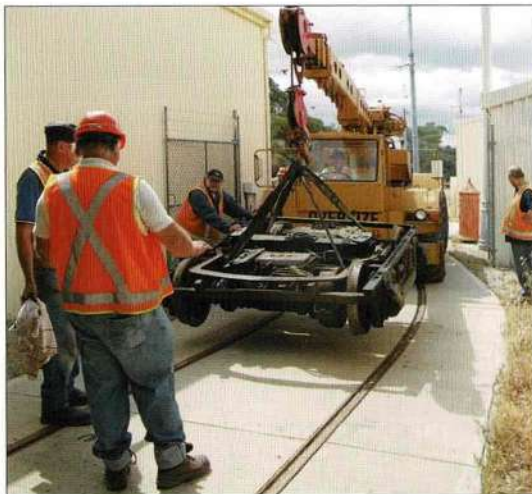
The replacement truck for SW2 426 on the pit road ready for installation after being transferred from the Engineering Shed by crane on 20 October. From left: Jack Kendall, Tony Kelly, Kim Freind and Graeme Eddington, with Noel Blackmore operating the crane.
