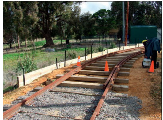
The replacement retaining wall near the south west curve. Jacqui Smith's small vegetable garden can also be seen near the small shed in the background ...not many tramways have their own vegetable garden!
