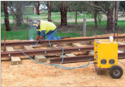
Kym Smith welds in the last section of outer rail to complete the curves behind the Car barn.
