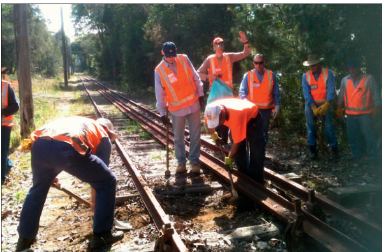
Volunteering as part of the Railcorp Community Challenge, a group of middle managers, engineers and project support staff tried their hand at replacing timber sleepers on the tram line north of Pitt Street. Ian Saxon
