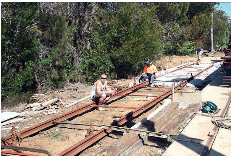
Reconstruction of the eastern track north of Pitt Street was well under way a week later. Martin Pinches
