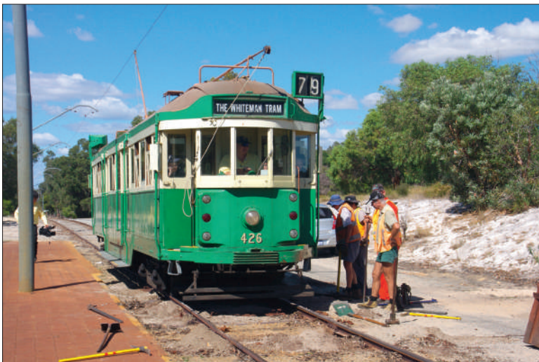
The track crew watch SW2 426 pass over a newly installed sleeper near the Village road crossing on 14 April.
