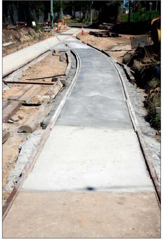
Two days later, the 'four-foot' of this track was concreted, with surplus concrete being used north of Pitt Street. The area to the left – the 'six-foot' - was concreted on 19 September.
