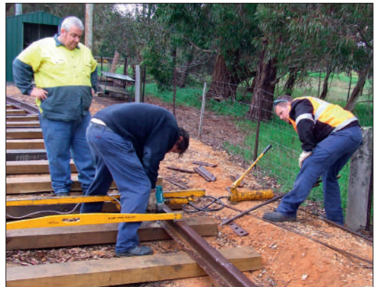
Anthony Smith driving home a dog-screw into the last of the sleepers on the south west curve as Alastair Reither supports the sleeper and Kym Smith observes the work. Jacqui Smith
