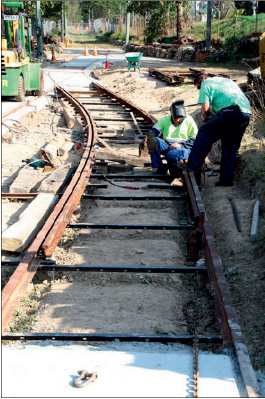
Welding steel angle iron sleepers and levelling of the new track curve just south of the Railway Square Waiting Shed on 12 September.
