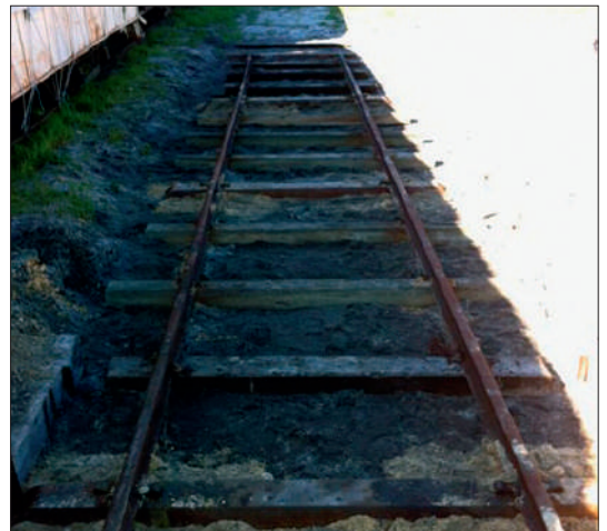
The completed first panel of track on the new truck storage road south of the Lindsay Richardson Carbarn on 21 July.
