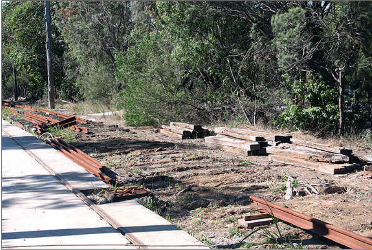
The eastern track north of Pitt Street being dismantled for reconstruction on 8 September. Martin Pinches
