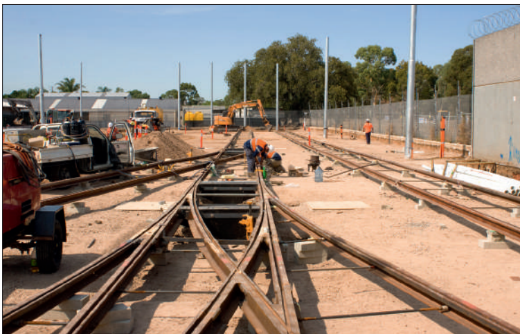
Construction of the special two-way turnout in the South Yard in February 2010.
