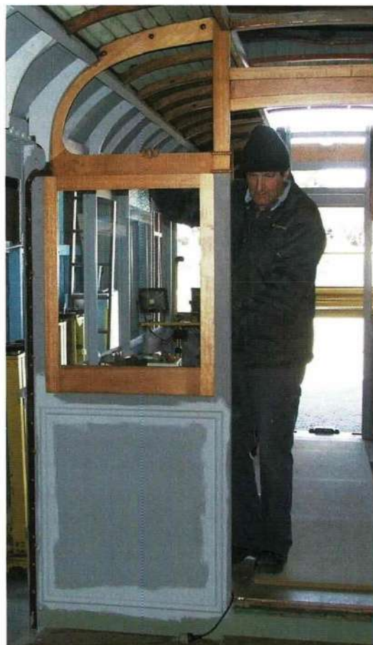
Test-fitting a replacement window sash to the drop-centre bulkhead of 792. Jacqui Smith
