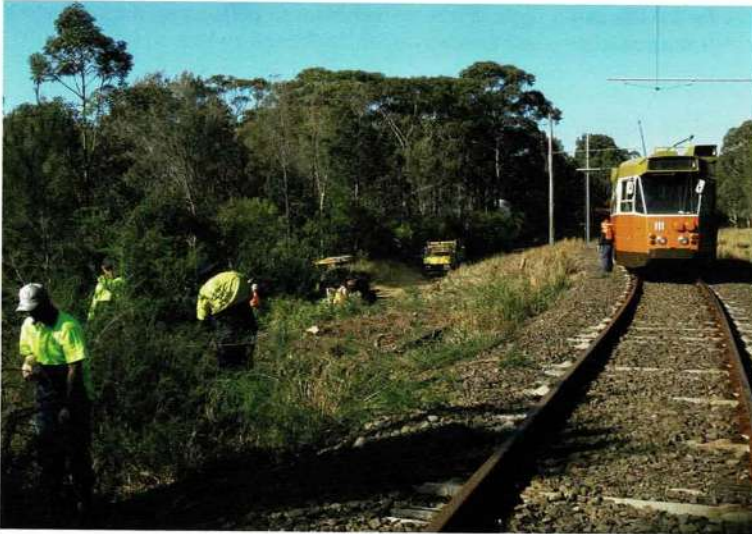
Tree and scrub clearing took place along the Royal National Park line on 30 June. The museum's new mulcher is at work in the centre of the photo.
