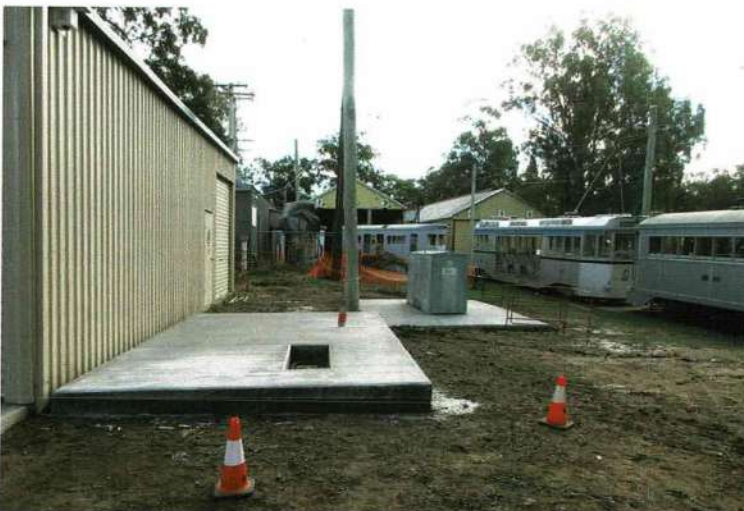
Concreting has been completed around the new substation. Trams have been removed from Depot No. 1 while re-roofing is underway.
