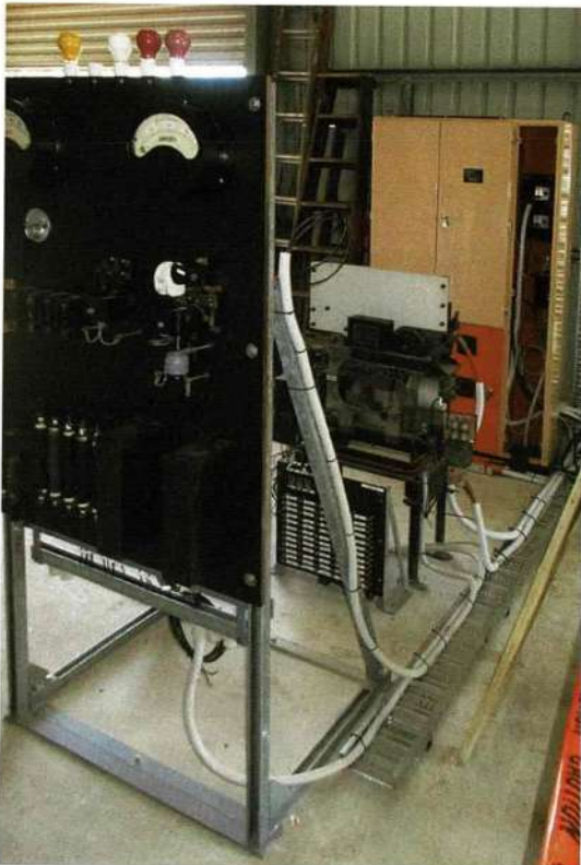
This view shows the Control panel (nearest camera), high speed DC circuit breaker and rectifier at rear.
