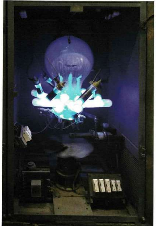
A view of the mercury arc rectifier just before it was closed down on Friday 29 June.
