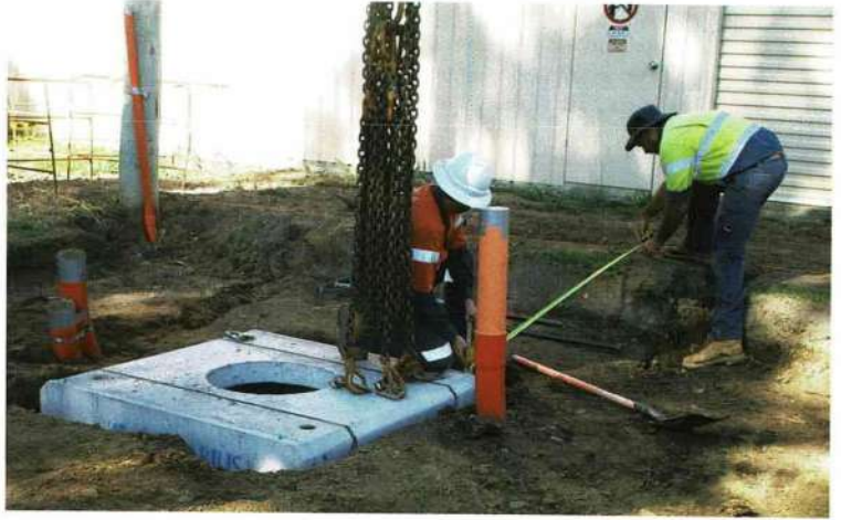
The large concrete culvert that is required under the padmount transformer before lowering into the excavated hole.
