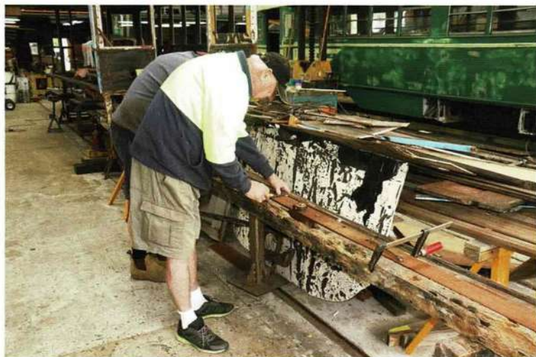
Warren Howlett and Terry Thomas preparing a new underframe timber for Melbourne cable trailer 589. Martin Pinches
