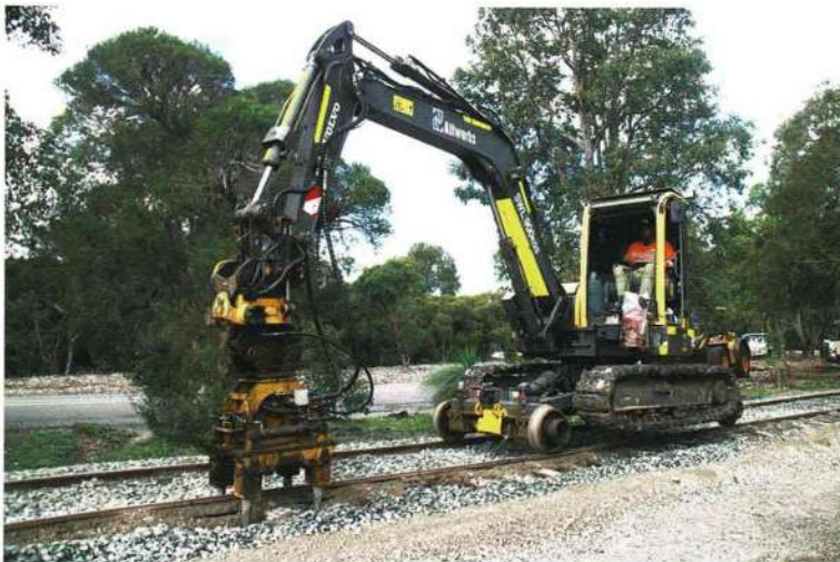
The Allworks steel sleeper packing machine completing its work on the newly-upgraded track between the previously-upgraded Village Junction Curve and the Village Junction terminus on 30 August.
