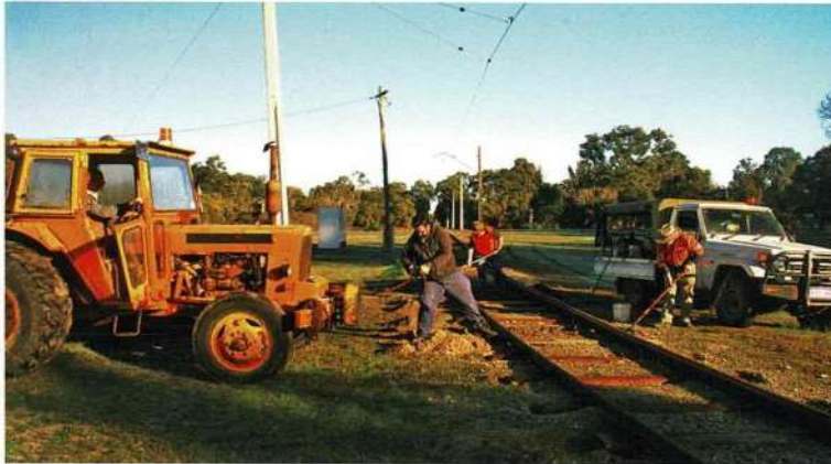
The track team replacing old timber sleepers at the western end of Farmgate Curve in the early morning on 16 June: Nick Tsiaglis attaches the sling to the next timber sleeper for extraction while Roy Winslow and Roy Daley (right) clear out the channels ready for steel sleepers to be inserted, after the timbers had been removed; Trevor Dennhardt is driving the tractor. Michael Stukely
