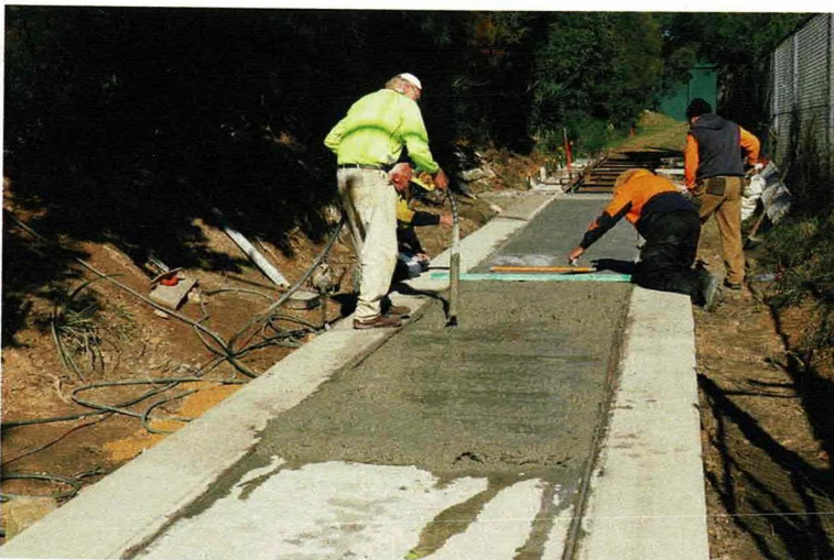
Finishing off a load of concrete in the 'four-foot' received on 10 July 2019.
