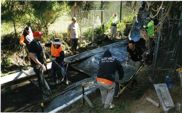
Receiving a load of surplus concrete on 15 June 2019. Many hands make the work load lighter. Martin Pinches
