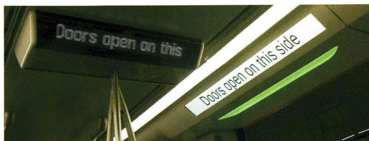
Doors Open on the Left / Right which changes to Doors Open This Side, then Doors Closing.
