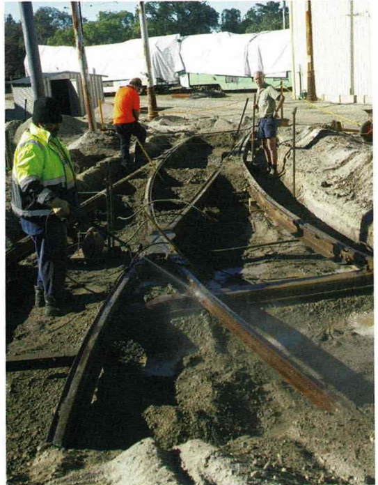
being extended, and the stop is being modified with access to be added for passengers with mobility restrictions.
