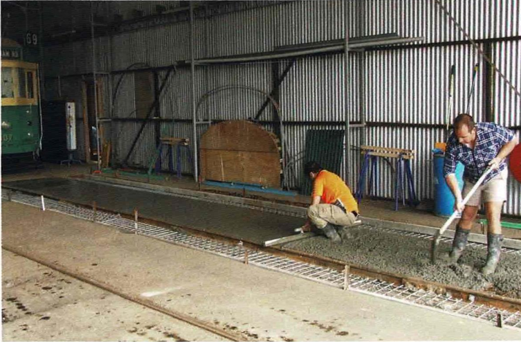
View showing the concrete pour under way on No. 5 road within the carbarn.
