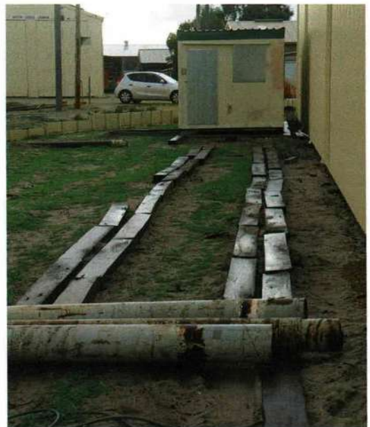
On 28 May, the building was moved along the sleepers laid on the south side of the Don & Laurie Tyler Carbarn, to its final position. The steel pole sections that had been used as rollers can be seen here, viewed from the east on 13 June. Michael Stukely
