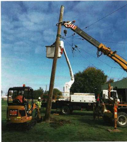
Digging out the base of the pole that really needed to be made vertical on 27 April. Paul Mong
