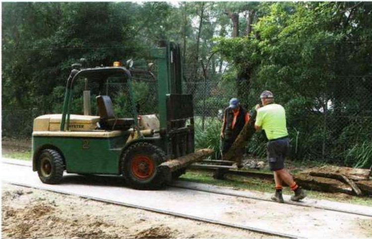
Old timber sleepers were removed on 9 May from the excavated track site using forklift No. 2. Martin Pinches
