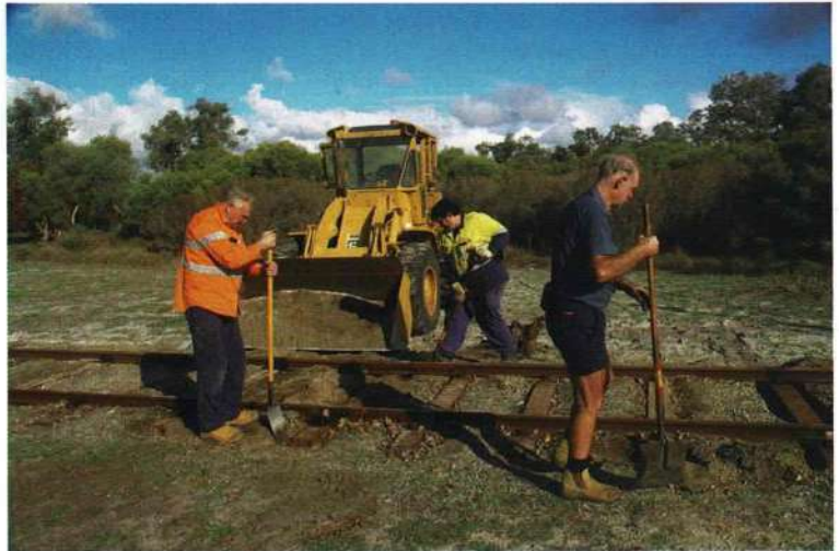
The track team hard at work on 13 June, packing the newly laid steel sleepers to the west of the Workshops Road level crossing: Terry Young (left), Nick Tsiaglis and Trevor Demhardt.
