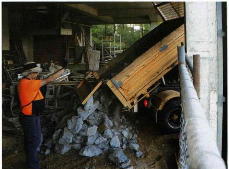
A truck-load of broken concrete is delivered to the ground floor of the YMCA building on 16 May. It will be used to lessen the amount of new concrete to be supplied. Martin Pinches
