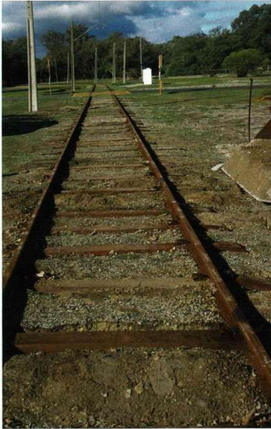
Steel sleepers were laid in May and June west of the Workshops Road level crossing. Michael Stukely
