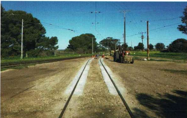
A new section of concrete track constructed by our contractors North East Demolitions on the approach to the Museum yard. 8 July 2020. Colin Seymour
