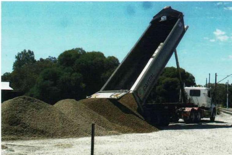
Delivery on 11 March of another 22 tonne load of road-base for spreading in the Don & Laurie Tyler Carbarn.
