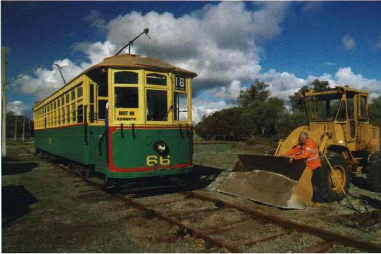
Terry Young watches as Perth E class No. 66 on a special trip passes through the track work site near the Workshops Road level crossing, on 13 June.
