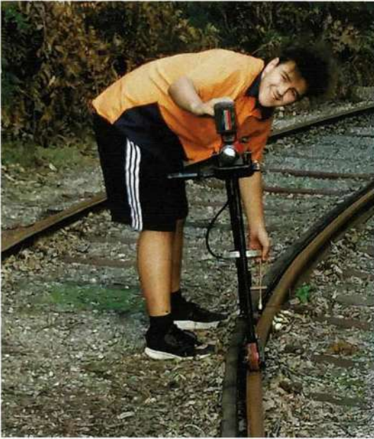
Aaron Antulov greasing the track on the Bennett Brook Culvert curve on 26 June. Allan Kelly
