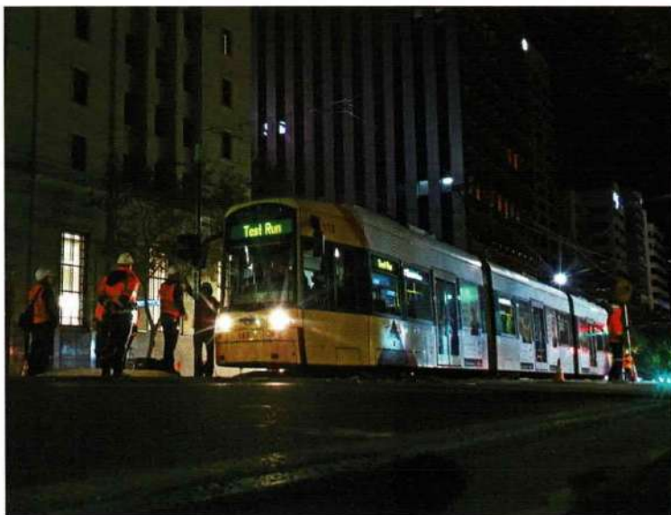
The King William Street / North Terrace Junction in the background with 113 on the first few metres running east along North Terrace on 4 June 2018. William Adams
