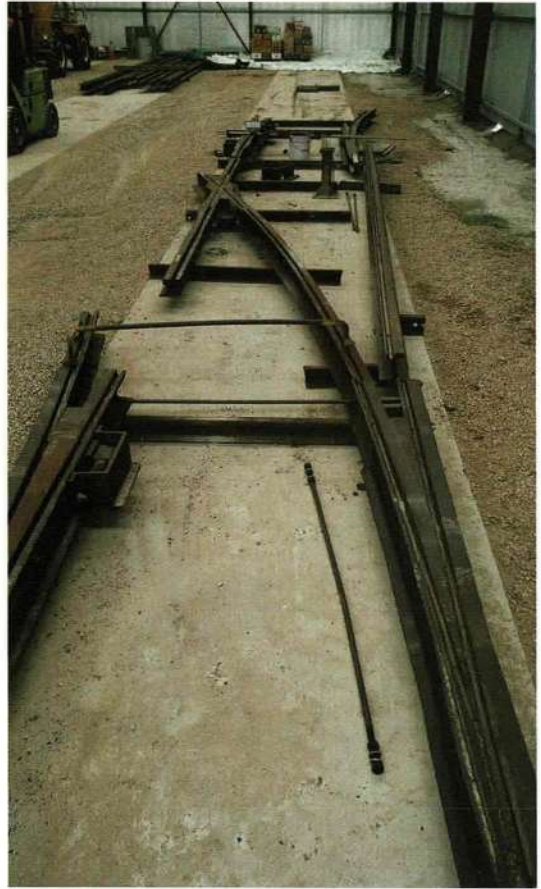
Point components for the new Don & Laurie Tyler Car barn fan being prepared and assembled inside the car barn by Brian Rourke on 15 July. David Brown
