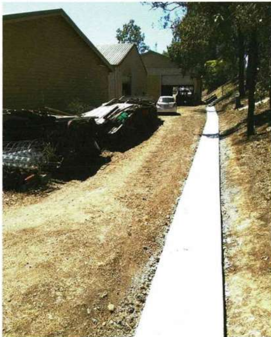
The concrete drain laid at the base of the slope above the Machine shop and store building. Peter Hyde
