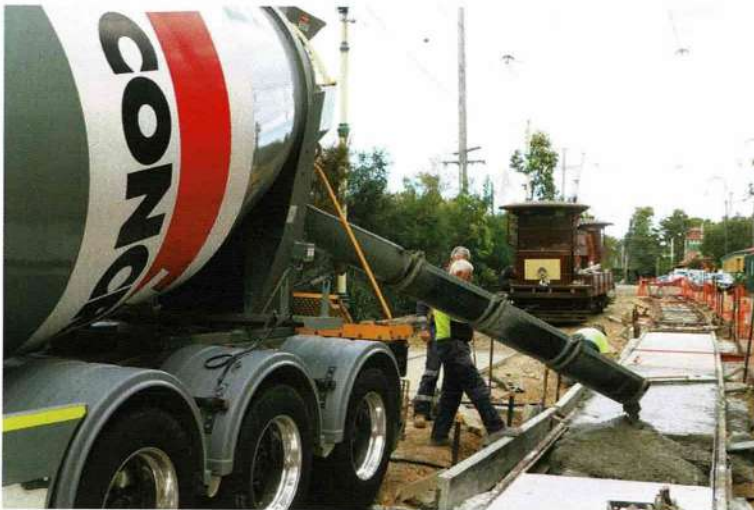
The first of two loads of surplus concrete arrived from Concrete on 19 August. A total of 3 cubic metres was received.
