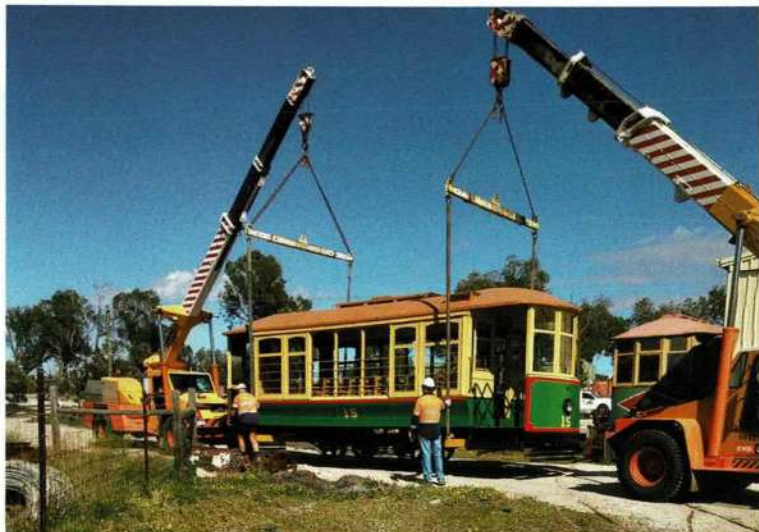
After being turned through 90 degrees using two cranes, B 15 is moved from the Lindsay Richardson Carbarn fan to the semi-trailer (out of view behind the tram) for loading on 25 September. The body of Perth E 64 can be seen alongside the carbarn at right.
