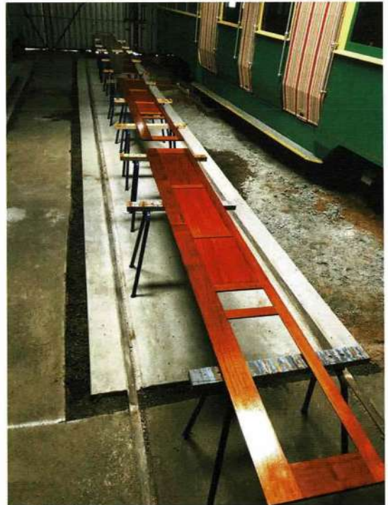
New saloon side walls in the process of being prepared for fitting into 792. Anthony Smith
