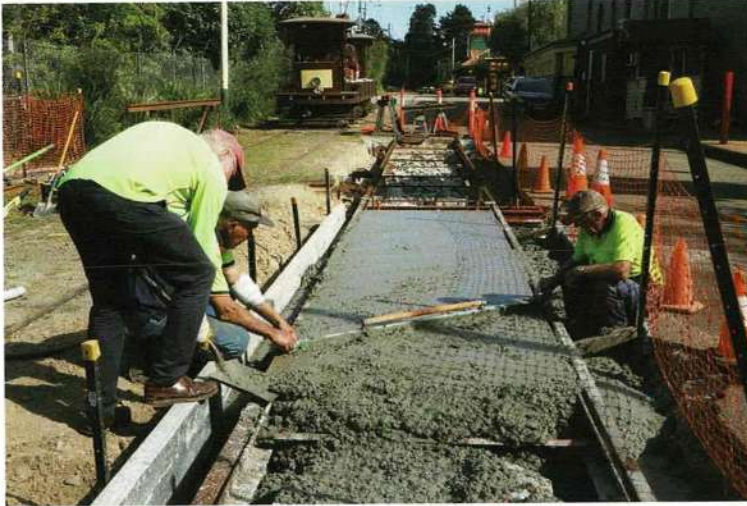
Andy Macdonald, Mike Giddey and Ian Saxon working on the track relay concrete on 16 September. Martin Pinches
