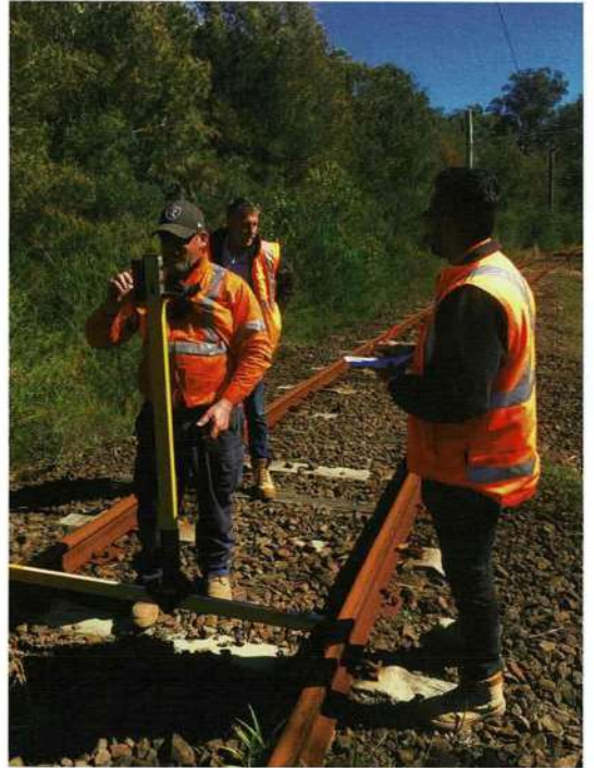
John Holland's staff taking preliminary measurements on 26 August prior to starting work on the Royal National Park overhead. Glenn Killham
