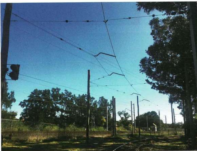
The additional pull-off spans using railway style pull off arms over the curve towards the highway level crossing.
