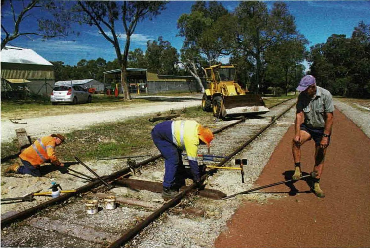
Installing a steel sleeper during remedial work on dropped rail joints near the Tractor Museum, south of the Village on 10 October: Terry Young (left) and Trevor Dennhardt (right) hold the sleeper in position while Nick Tsiaglis attaches the rail fastenings. Michael Stukely
