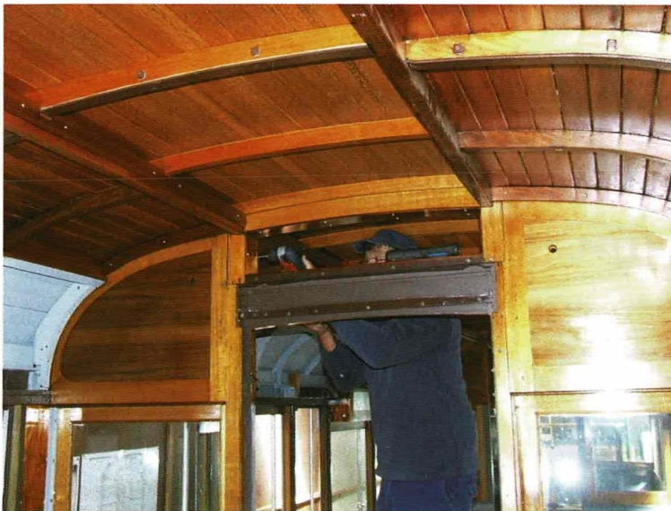
Cover strips being fitted to the archway over the No. 1 end saloon door. Daniel Edwards
