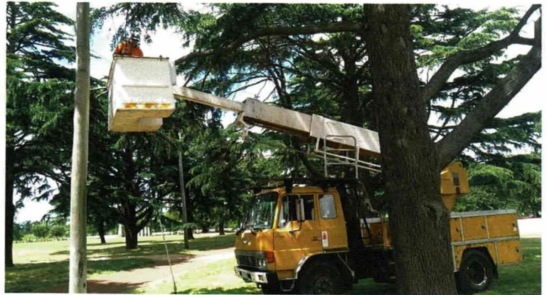
Maintaining the overhead on the access track, manoeuvring around the trees on 17 November 2020 Sam Boon
