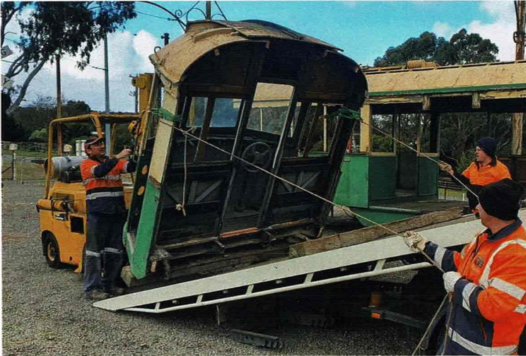
Cab from W5 826 being loaded onto a tilt tray on 4 June 2021 after being sawn off the end of the original tram behind. Left to Right is Tony Smith, Alastair Reither and Paul Mong.
