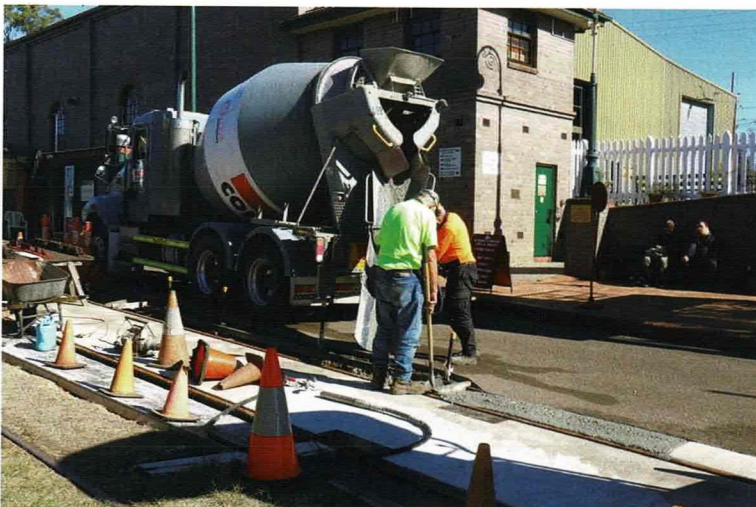
Concreting the last of the western track in Tramway Avenue on 26 May 2021. Martin Pinches
