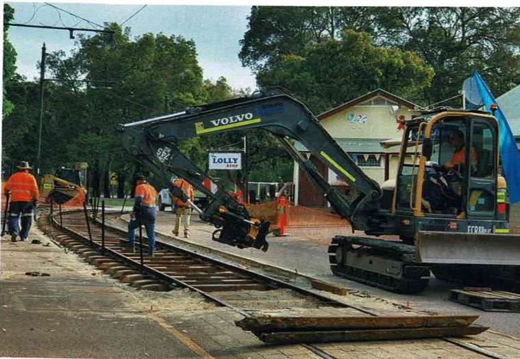
Stage Two of the Village Mall track upgrade is well under way on 23 April, with Allworks workers adjusting the alignment of the new track ready for concreting. Michael Stukely
