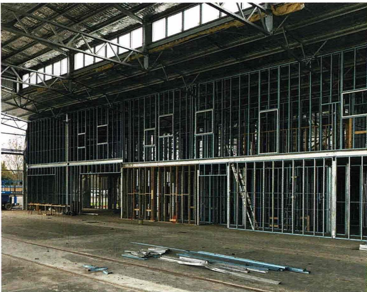
View on 22 June 2021 looking at the future Exhibition Room, kitchen and store on the ground floor and the Collection / Archives store and offices on the second floor.
