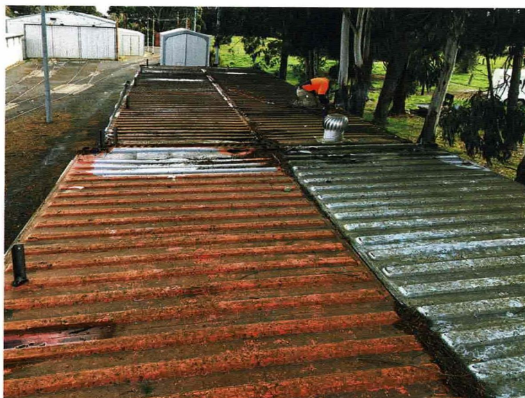
Brackets for roof beams being welded into position on former shipping containers.
