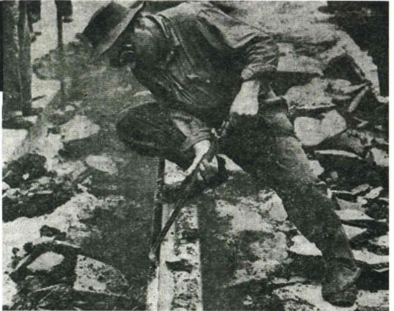
Workmen are constantly employed ripping up Sydney's disused tram tracks and repairing the streets afterwards.
