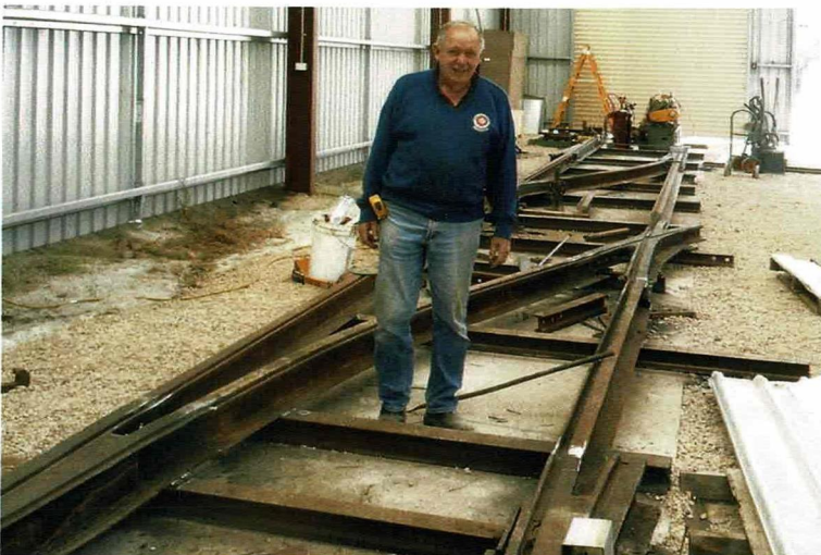
Brian Rourke viewing his preparatory work for turnouts to be installed in the main line approach to the three roads leading to the Tyler Car barn. 7 July.
