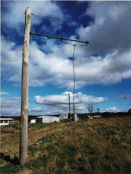
A view looking towards the museum showing the trolley wire cut.
